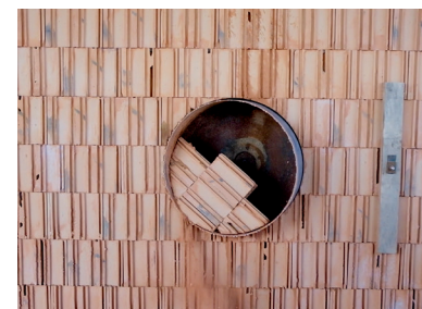
Drilling a round window through the wall in the container park in Luchtbal
